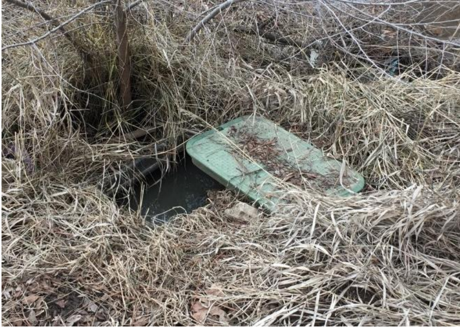
Figure 4: open Valve Box
