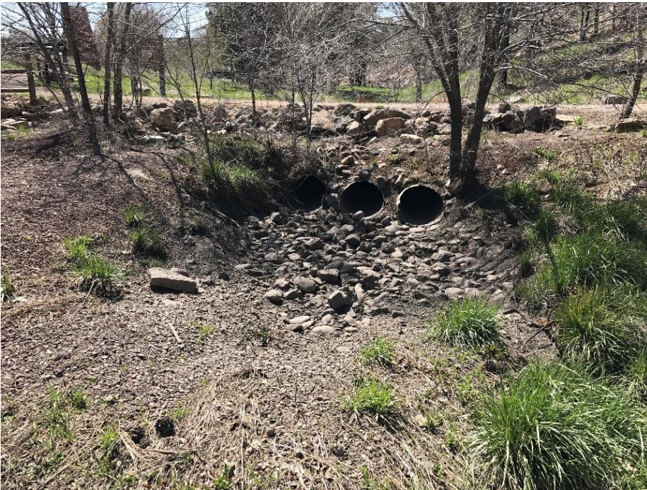
Figure 5: Deep Scour Pool
